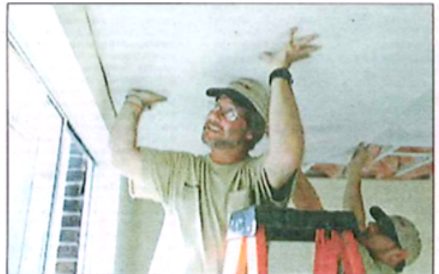
Sheldon Yellen, the CEO of Belfor, the world's largest disaster-restoration company, goes undercover and becomes frustrated while struggling to hang drywall at a construction site.
